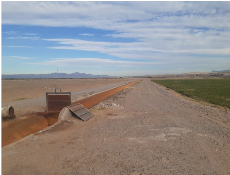
Figure 8: Mohave Valley Irrigation and Drainage District Flood Gate
