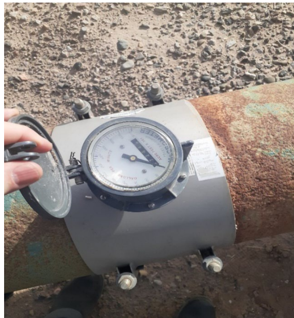
Figure 7: Mohave Valley Irrigation and Drainage District Flow Meter
